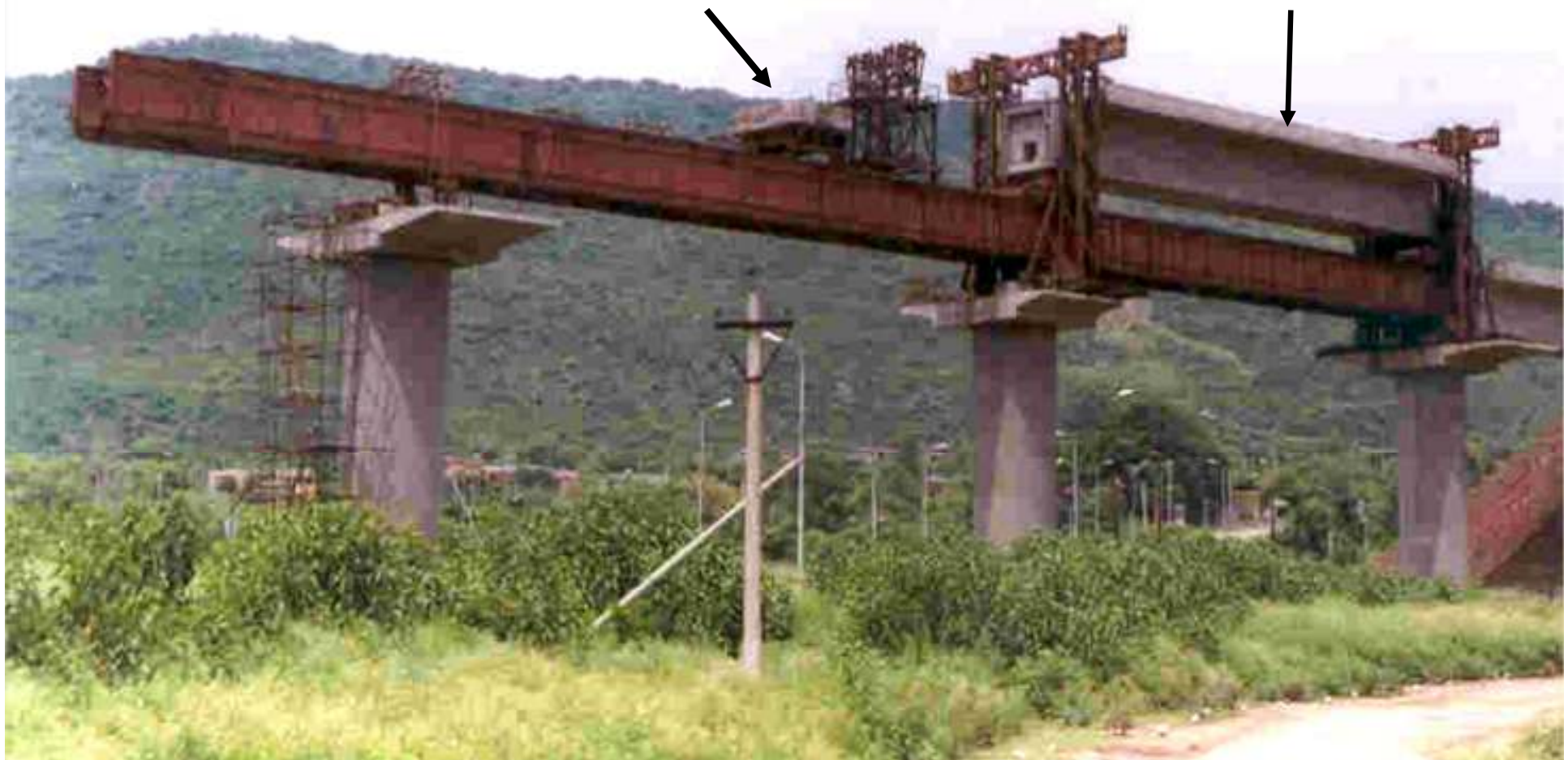
JURL: VIADUCTE18 LIFTING OF PSC GIRDER IN ORDER TO MOVE LAUNCHING GIRDER FORWARD
